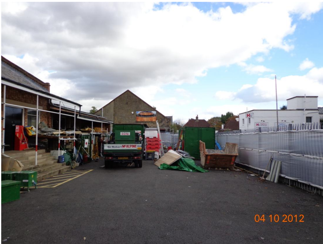
Looking north-west from within the application site capturing the rear elevation of Ladbroke House, No 60 Highbury Grove and the buildings (and extension) to the rear of No 58 Highbury Grove to be demolished
