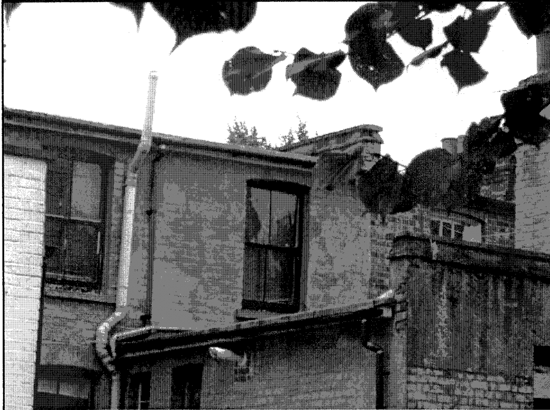
View from rear garden looking towards 91 Harberton Road to the south west.
