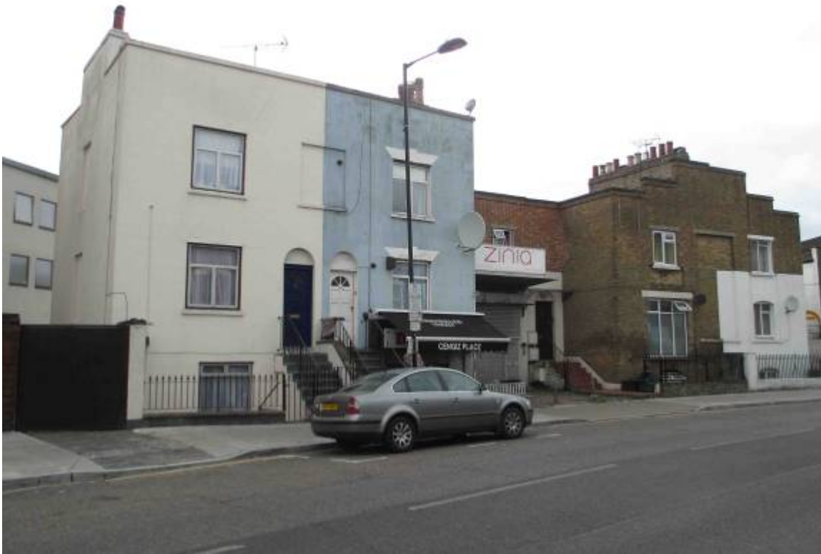
Figure 41 Numbers 45 and 47 Green Lanes (left of picture) and numbers 49 and 51 (right). Note that these buildings date from the 1820s/30s but have been extensively altered.
