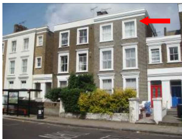
Figure 43 Numbers 48 (right of picture), 50 and 52 (left) Mildmay Park. Note that the principal front elevation to number 52 has been rendered over. The mortar to the brickwork of number 48 has also been poorly applied and finished (arrowed).
