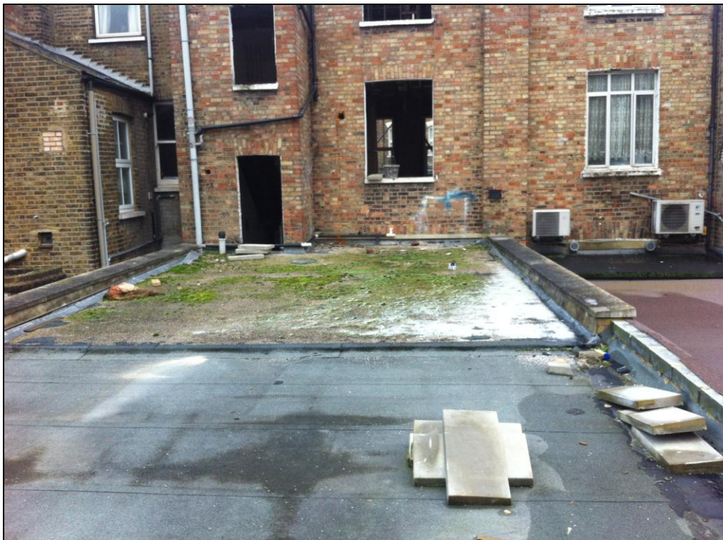
On top of the ground floor rear extension looking toward the rear at first floor level
