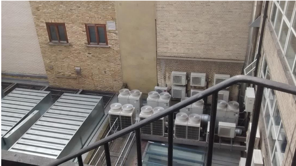
Image 2: View of the Rear of the building from existing fire escape including existing A/C plant and plant serving data centre
