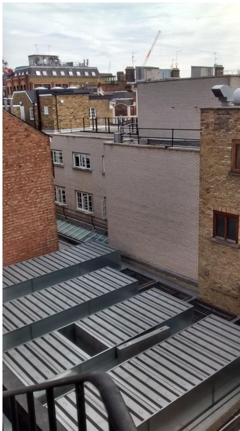
Image 3: View of Existing Data Centre Plant and part of rear façade of 24 Epworth Street
